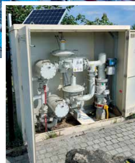
Self-sufficient installation for measuring the gas quality
